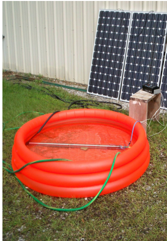
Solar pump and panels.
